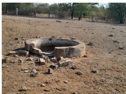
Figure 15. Collapsed water trough at Lusenga Dip Tank
