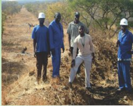
A standard fire guard constructed at the Fire project in Woodrich farm of ward 30 in Kwekwe district. The fireguard stretch is 5 Km
