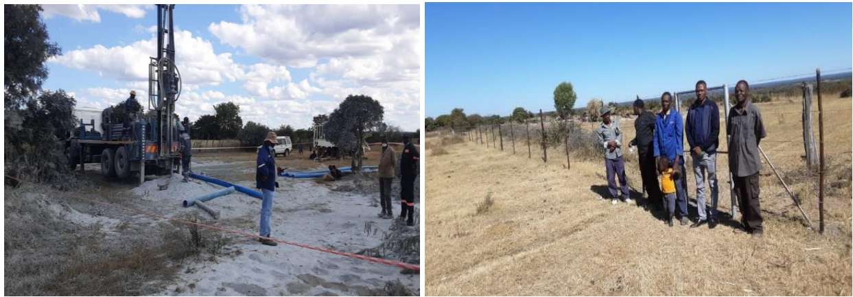
Plates 18 and 19: Borehole Drilling and Casing at Matambo Wetland And Part Of The Perimeter Fence Used To Protect The Wetland Core -Gweru(25/04/2022).
