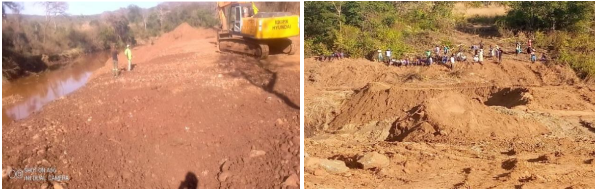
Plate 7.2: Rehabilitation In Progress On Mutebekwi River By ENR Resources In Shurugwi (26/07/2021) And (Right) Community Protests Against Lightweight Investments Which Blocked The Nyagwi River (Goromonzi) Where Rehabilitation Was Done After Agency Intervention (14/05/2021).
