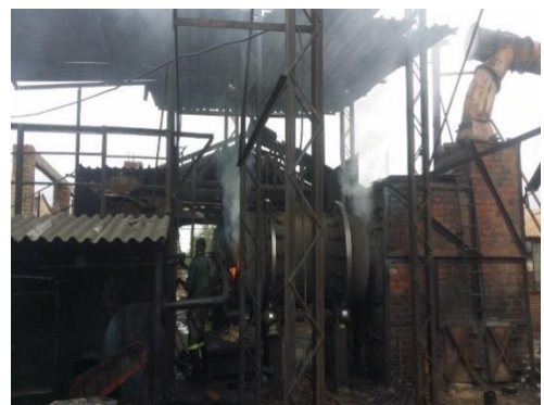
Plate 2.1: Fugitive furnace emissions at Central African Batteries (01/03/2021).
